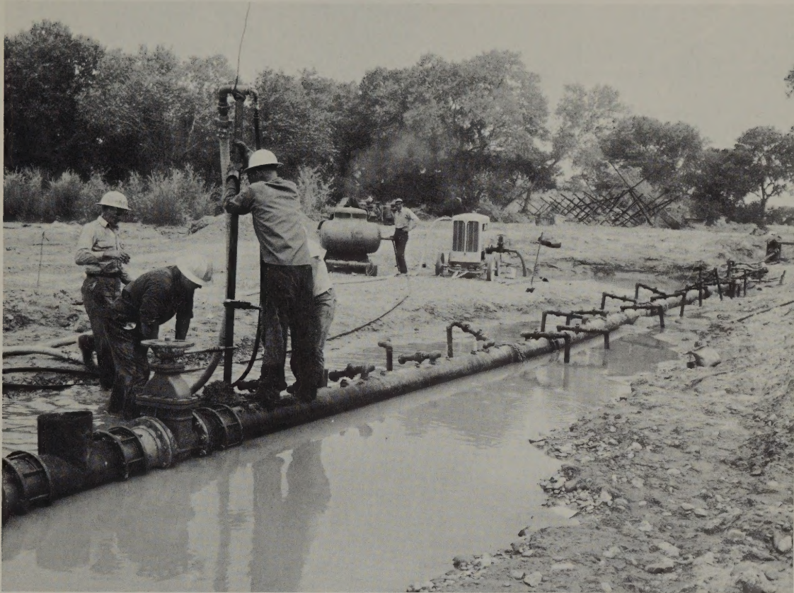
Preparing to build an irrigation structure, these engineers pump water from the ground to dry the foundation.
